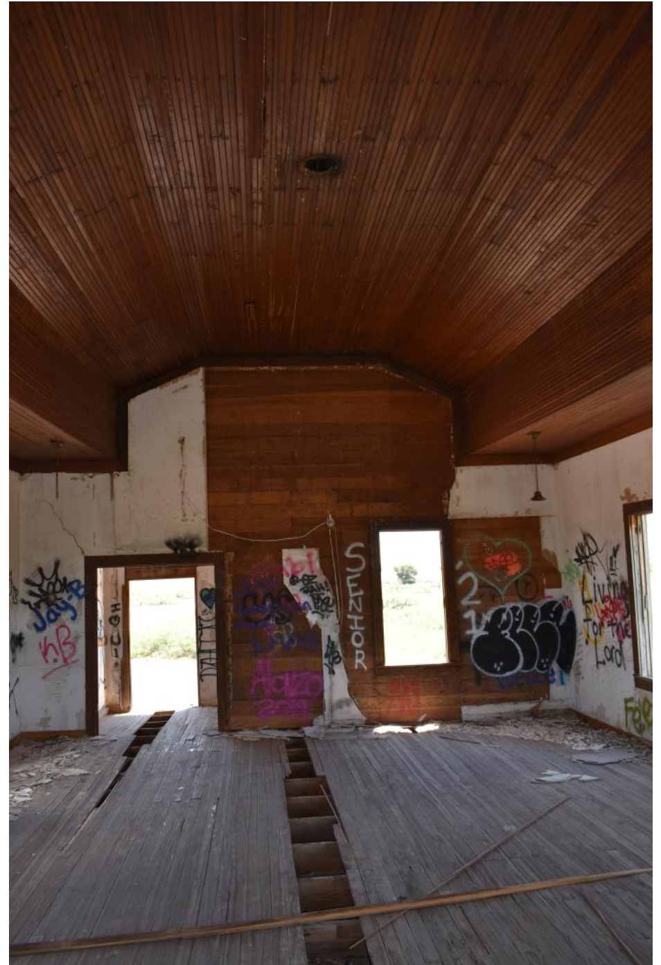
Looking towards the south end of the interior, front door to the left.
