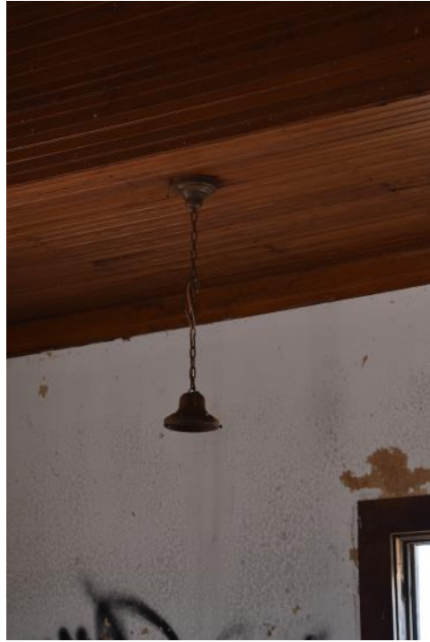
Two of the last light fixtures after the church gained electricity in possibly the late 1950s.
