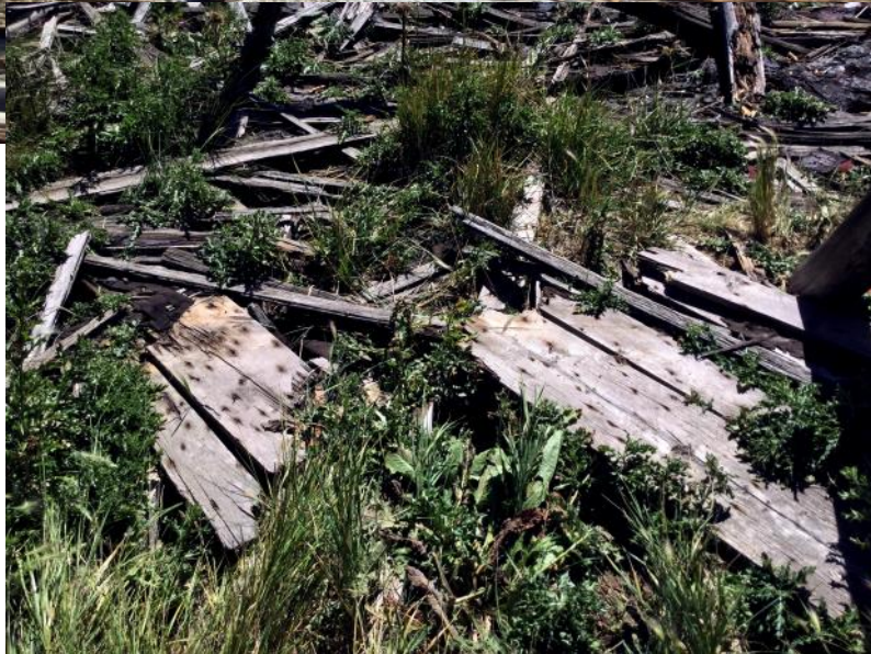
You can see the floor boards running diagonally across the floor joists here near the front door.
