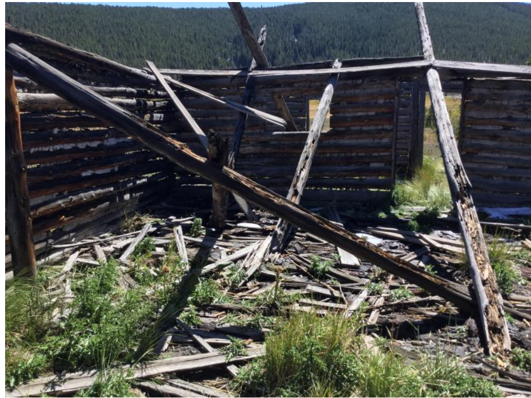
The walls seem more structurally sound, but the roof and the floors are completely gone.
