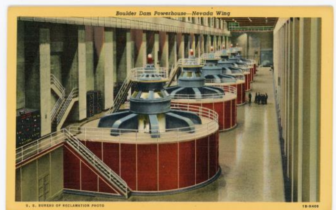
Boulder Dam Powerhouse—Nevada Wing
