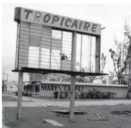
After Hurricane Andrew, 1992 Photo by: Robert A. de Stolfe
