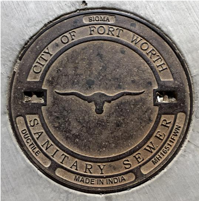
Why is this manhole cover made in India??
