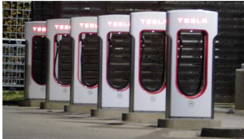
Six Tesla charging stations behind the Tower Station.
