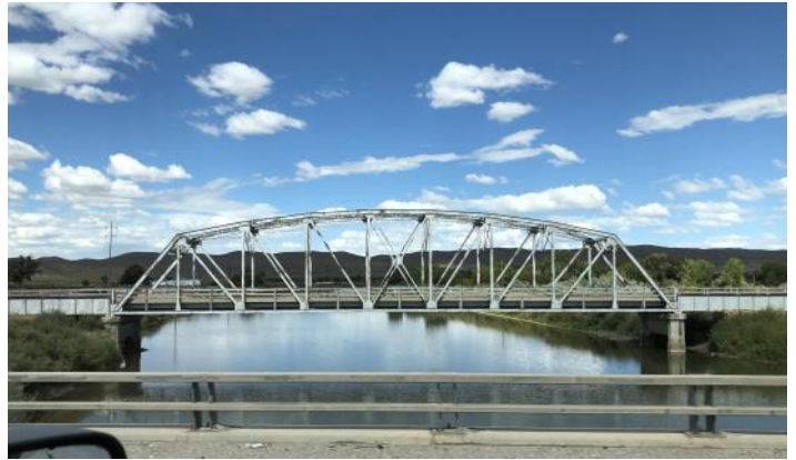
Saw this metal truss bridge while on I-80 in Wyoming. It is the Old Highway crossing over the North Platte River near Fort Steele.
