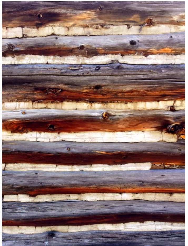
Being a log cabin, the gaps between the logs would have been chinked. Whoever built this cabin had a very interesting technique to hold the chinking in place!
