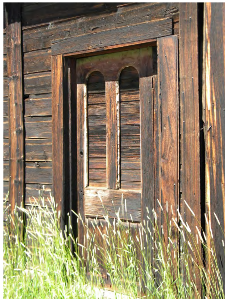
The style of this door suggests that this house might have once been nice. The two arches in the door likely would have been glass.
