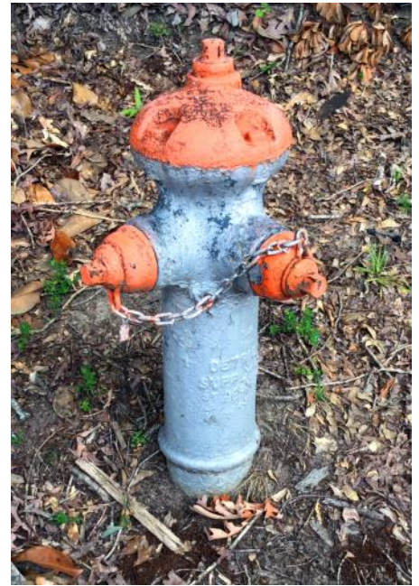
Old style hydrant (modern painting).
